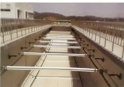
Sea water desalination facility
