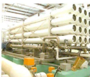
Low energy seawater desalination plant -Hawaii Energy Saving R/O
