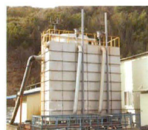
SAB(Shingang Advanced Biological Reactor)
