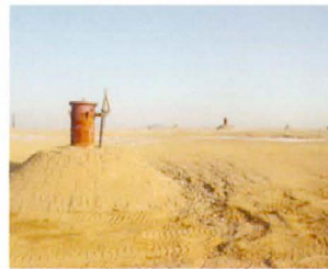
Landfill gas collecting pipe
