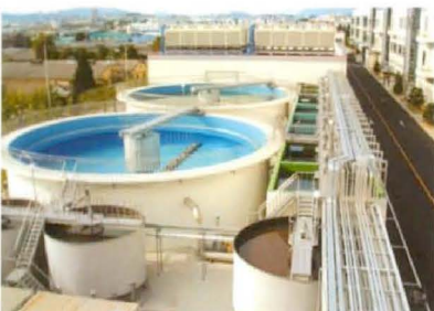
| WASTEWATER TREATMENT SYSTEM (24000m 3 /DAY)
