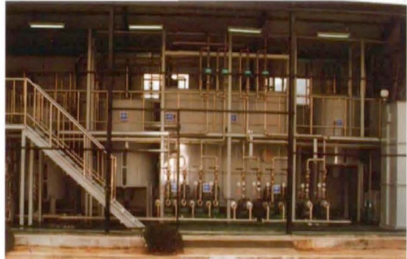
Site : Uijeongbu Environment Affairs Agency Use : DBS Sewage Treatment Capacity : 89~112m 3 /day HRT : 10.5hr
