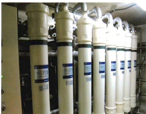
| Dual water membrane filtration system in Intercontinental Hotel, COEX
