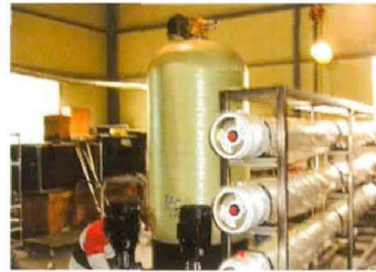
RO(Reverse Osmosis) SYSTEM
