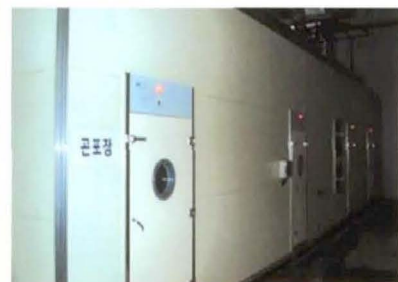
| EG Clean Air conditioner
