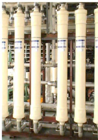
| Commercial plant which will be established at the Yeongdeok Jipum Purification Plant
