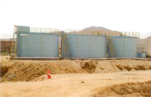
Site : Gae-Seong City, N-Korea Material : Epoxy Coating Use : Waste-Water Treatment System Capacity : 600 m 3 /day Date : 2005. 06
