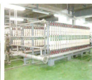
Waste water treatment and water re-use system SEVERANCE HOSPITAL water re-use system (dual water supply)
