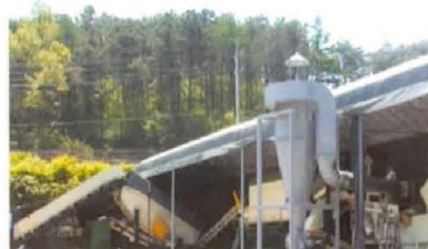
An overall view of FORCEBEL-MBT System in the company
