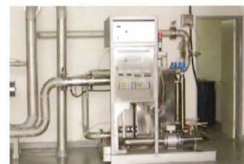
| UV Disinfection System
