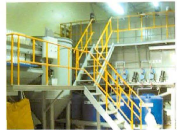
Physical chemistry treatment facility
