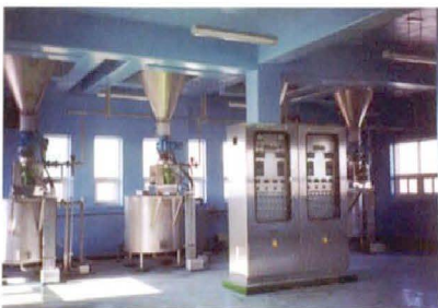
Clean water processing facility
