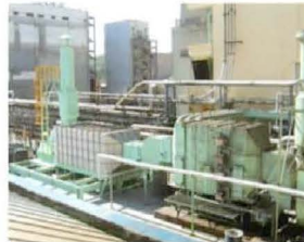
Domestic vinyl wallpaper manufacturing factory - D.O.P/OIL MIST
