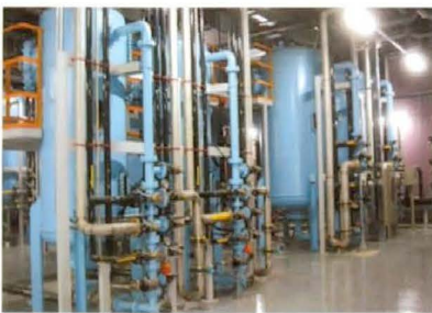
| DEMI. WATER SYSTEM(1320m 3 /DAY)
