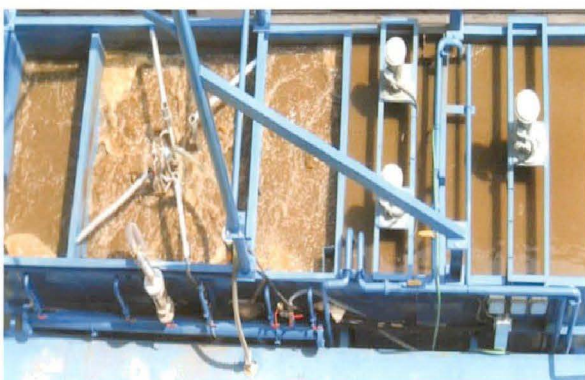
| MBR Plant for waste water treatment
