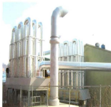
Heat Switchboard (For Organic Solvents)
