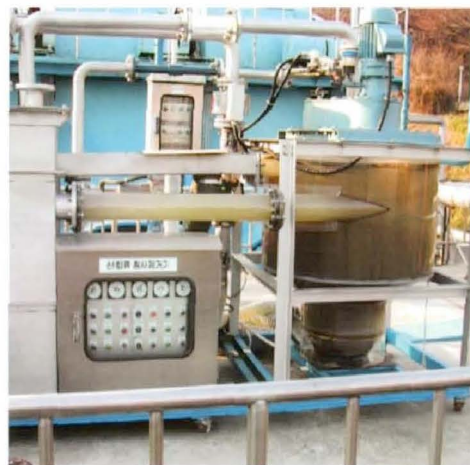
| Spiral flow grit remover
