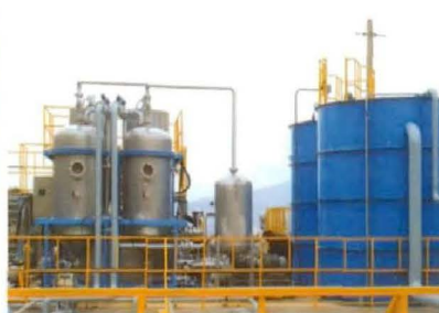
Pre-coated filter supplied at the tunnel excavated water disposal facility
