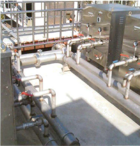
Wastewater Treatment Device
