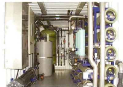
Waste water processing facility
