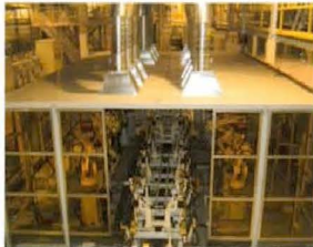
Automobile Body Factory of the Europe Office - WELDING FUME/GRINDING dust collector
