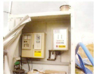
GBS gas analysis and control panel
