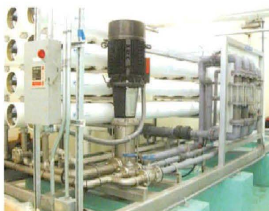
Reverse osmosis system
