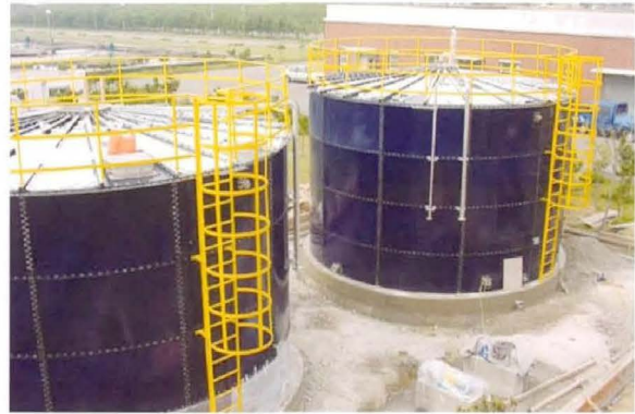
Site : Ul-San City Use : High Solid & Chemical Storage Facility Capacity : 160 m 3 X 3 units Dimension : \varnothing 6.8m X 4.6mH Date : 2003. 05
