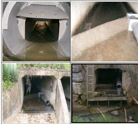
Fig. 1. Namchen bridge NPDR and flow meter.
